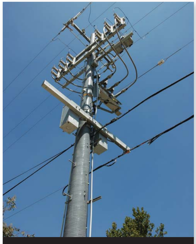
This composite-pole top on the "Circuit of the Future" has a vacuum recloser and bypass switches. (Photo by Kevin Coates.)
