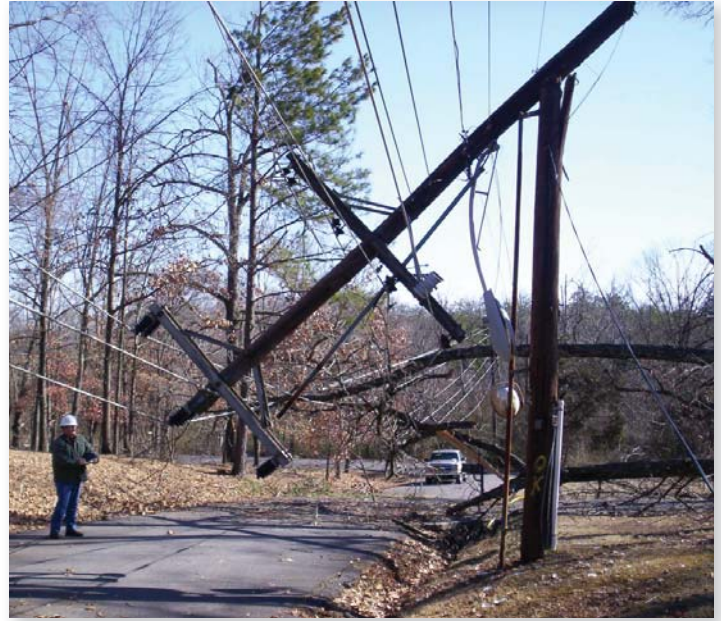
Winston Chambers, a contract engineer with Patterson & Dewar Engineers, assesses damage to a double-circuit joint-use wood pole.
