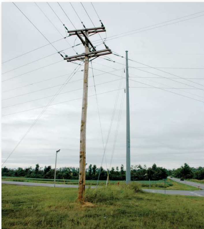
This wood pole was used to replace a steel pole that was damaged by the ice storm because there were no composite poles in stock.
