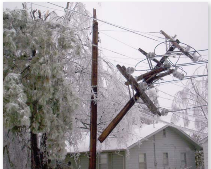
An extreme icing load caused this double-circuit double-deadend wood pole to snap.
